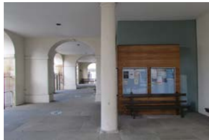
Current screens to entrance foyer do not allow view to the inside from some angles
