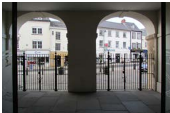
Configuration of existing railing and gates, while performing a necessary function, hinders open access to the loggia
